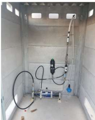
1. Supply Room Refrigerant transfer pump (RTP)
